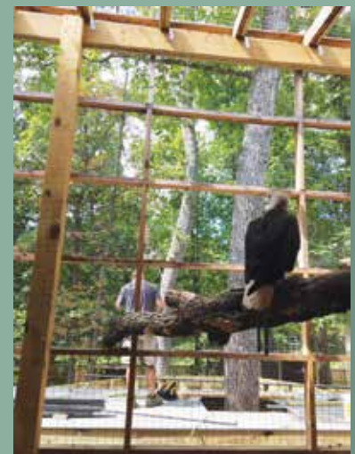
Jefferson monitoring the construction of the Observation Deck. Photo by Jessica Andersen
